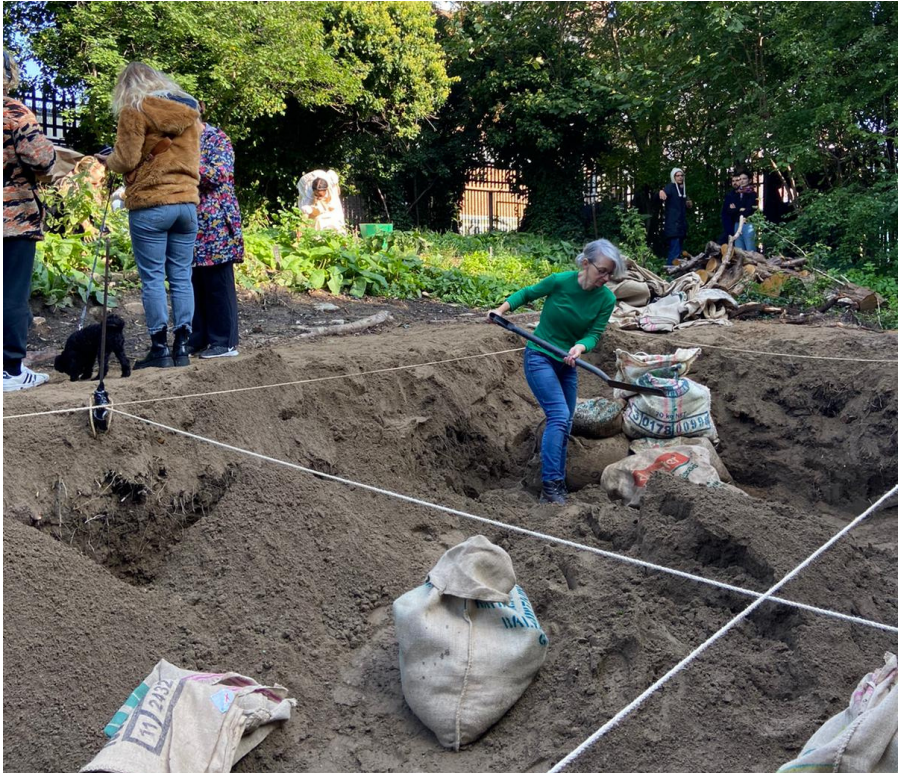
Filling hessian sacks with recycled soft sand to make building blocks for the corners of the pond. Photo: Michael Smythe.
