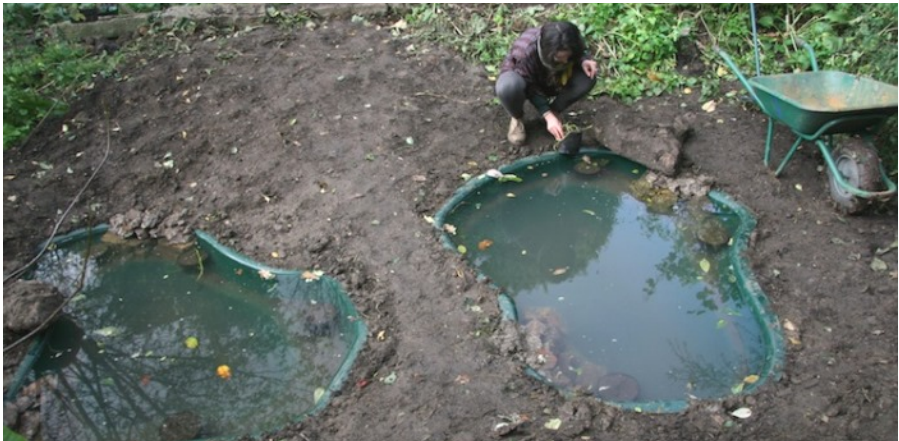
Installation of modular ponds at the Bethnal Green Nature Reserve. Photo: Nomad Projects.
