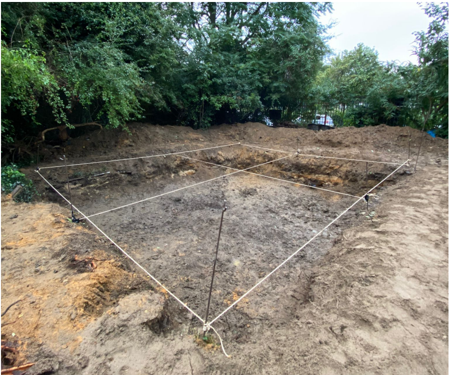
Metal stakes and rope mark the dimensions of the new pond on the excavated wetland site. Photo: Dimuthu Meehitiya.
