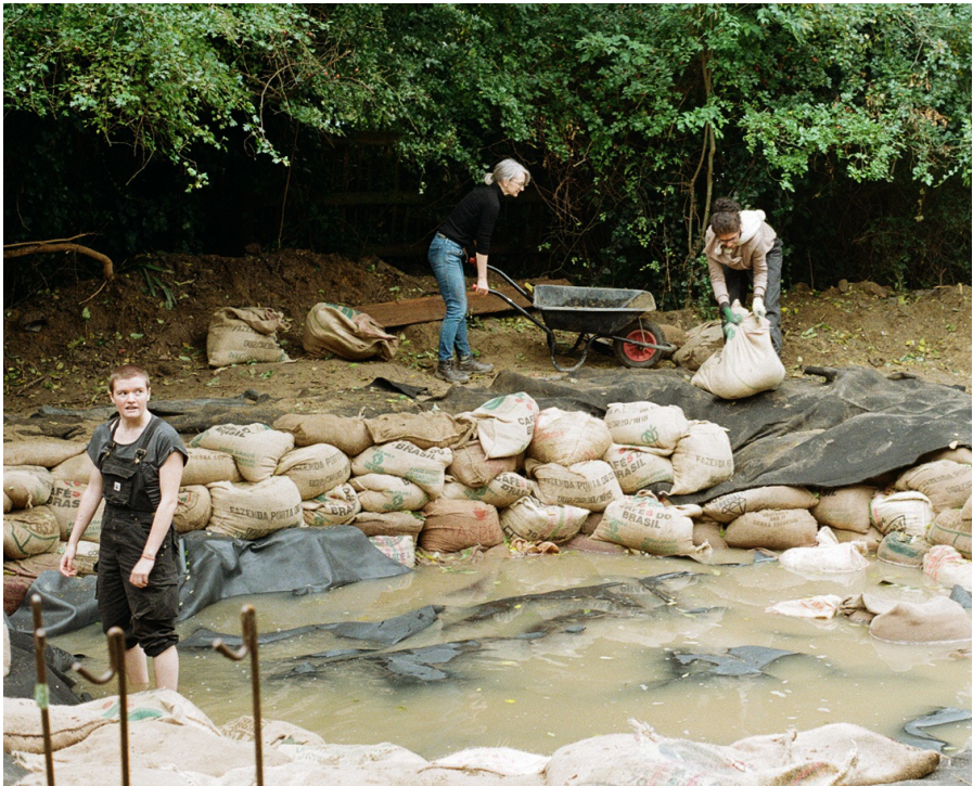
Creating sloping banks and shaping the pond with earth and sand-filled hessian sacks.
